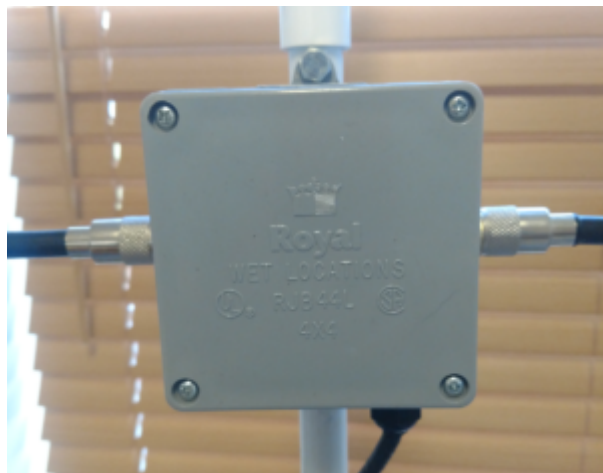
Outdoor Utility box.
