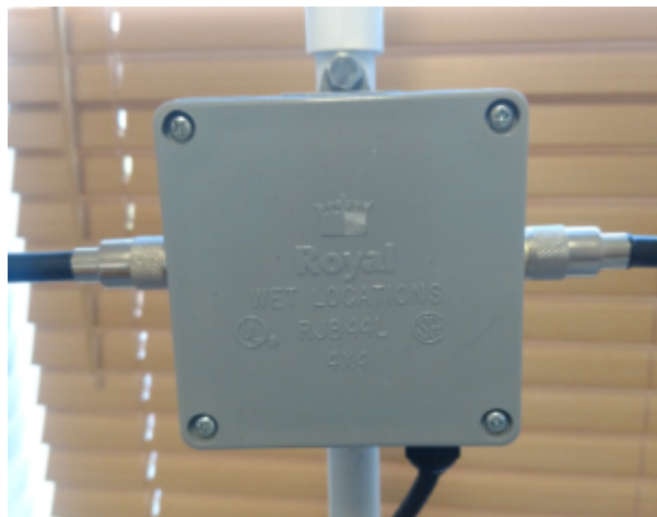
Outdoor Utility box.
